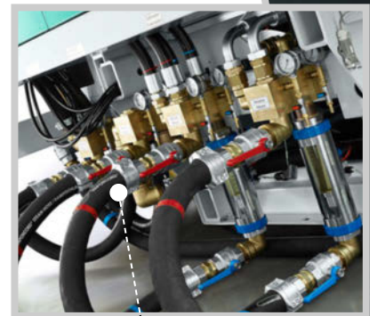
Effective cooling: supply lines with large cross-sections.
