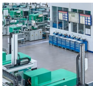
Host computer system Energy measurement of the entire production
